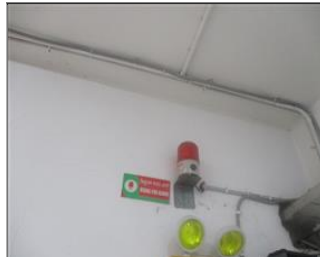
External photo(s) of the production unit(s) Visual fire siren.JPG
