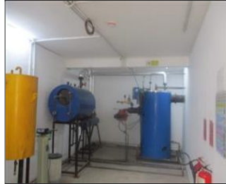
External photo(s) of the production unit(s) Boiler section.JPG
