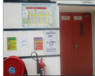
External photo(s) of the production unit(s) Fire rated door.JPG
