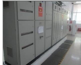
External photo(s) of the production unit(s) Electrical Distribution board.JPG
