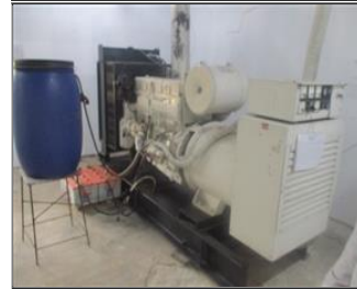
External photo(s) of the production unit(s) Generator.JPG
